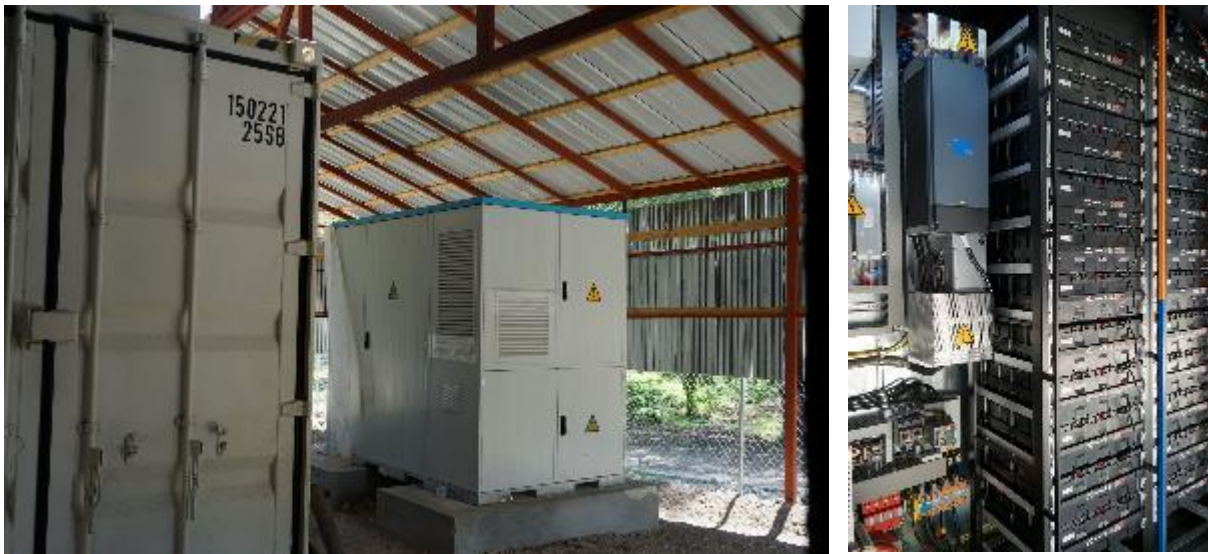
Figure 7: The BESS setup from the outside and the inside.
