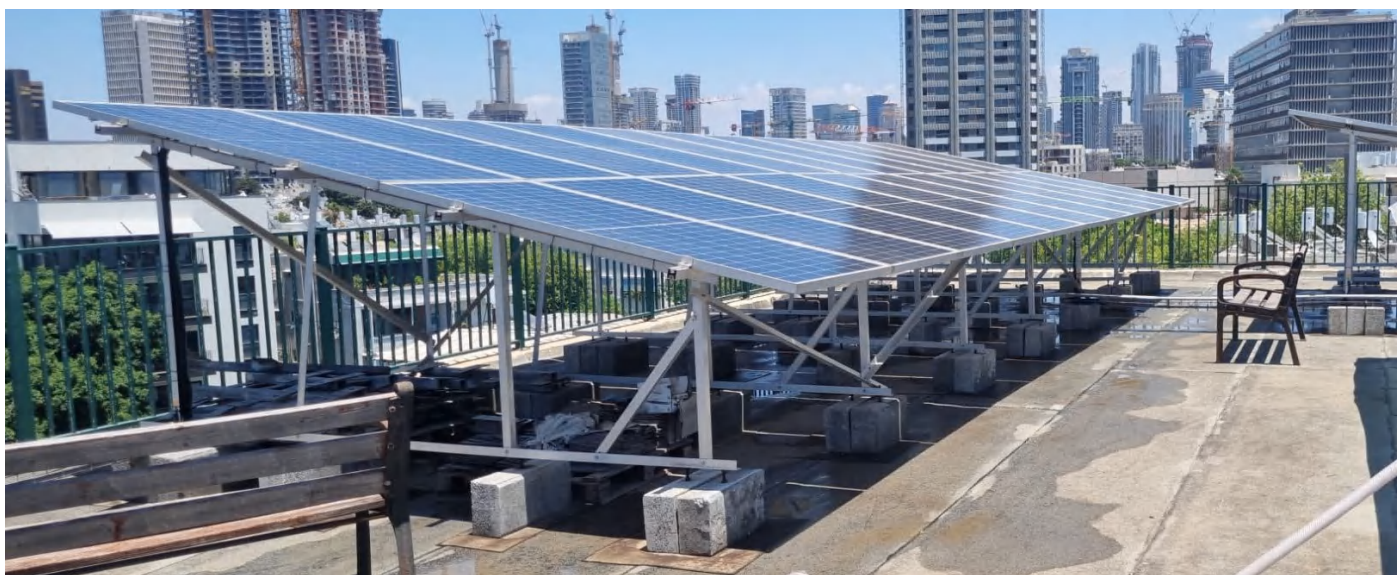
Figure 22: Urban rooftop PV installation in central Israel, highlighting the integration of solar energy into densely built environments.
