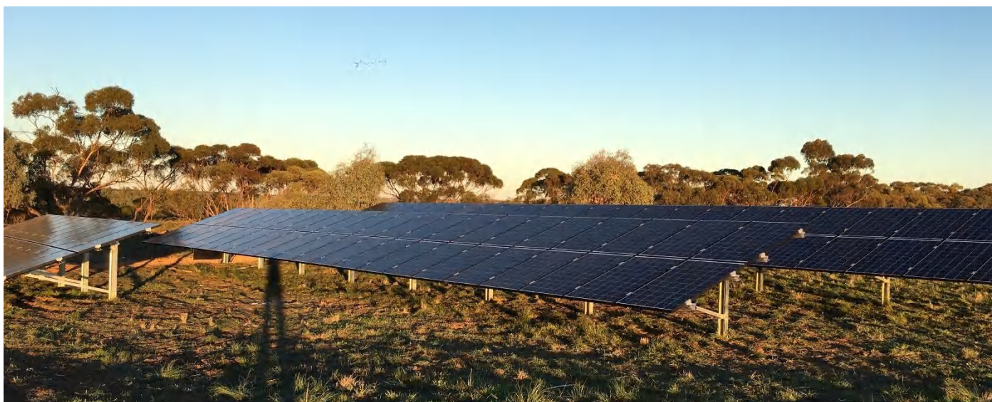
Figure 2: 30 kW ground mount install in regional Australia. Photo courtesy of Tindo Solar, Australia's leading solar manufacturer.
