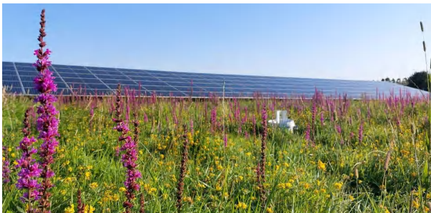
Figure 38: Picture Eco certified solar park, courtesy TNO.
