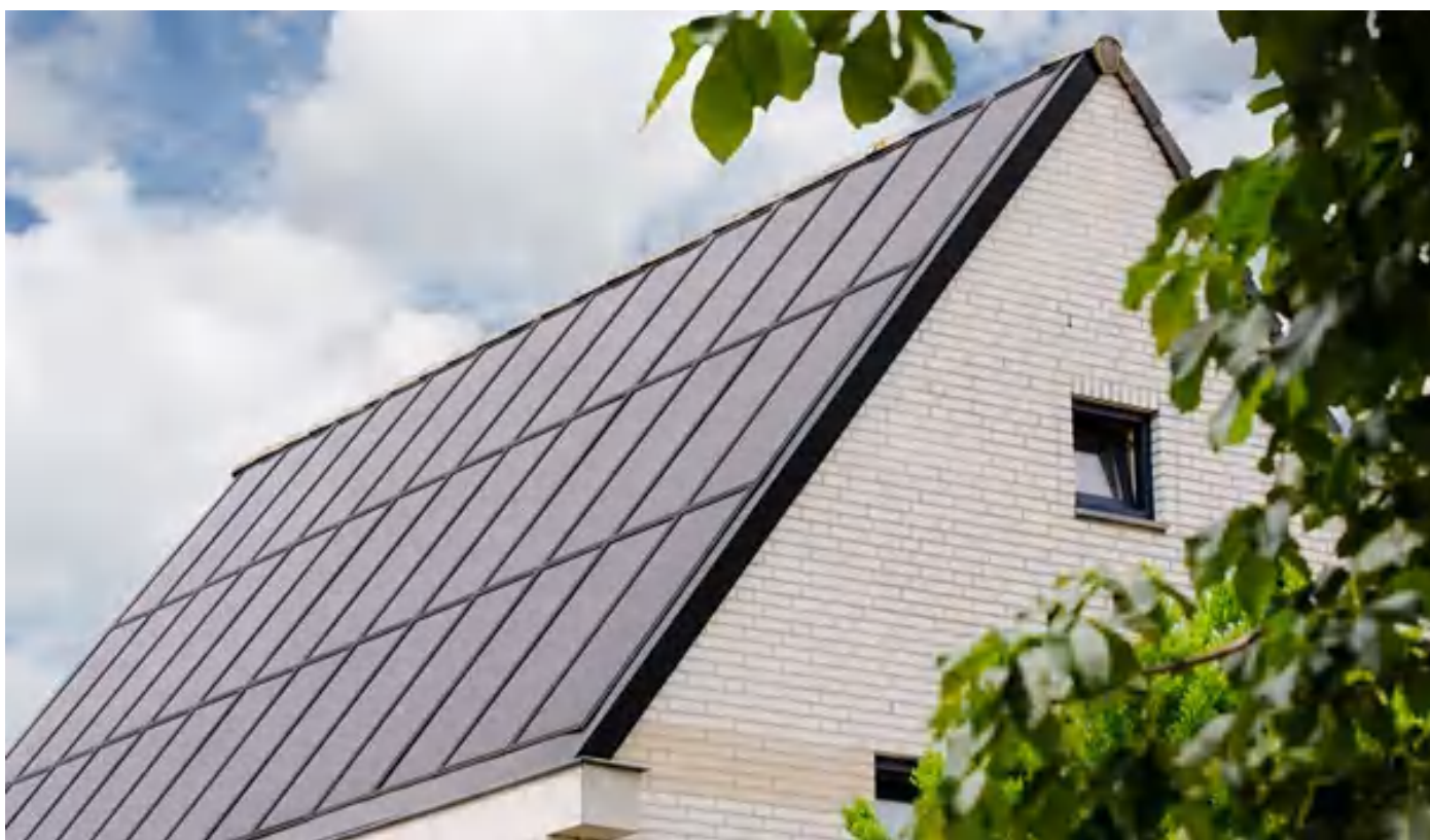
Figure 37: Solar integrated on Roof, image bank RVO.
