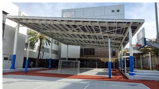
Figure 21: Solar canopy over a school sports facility in Israel, reflecting national efforts to promote PV deployment in public buildings and maximise dual-use of urban space.
