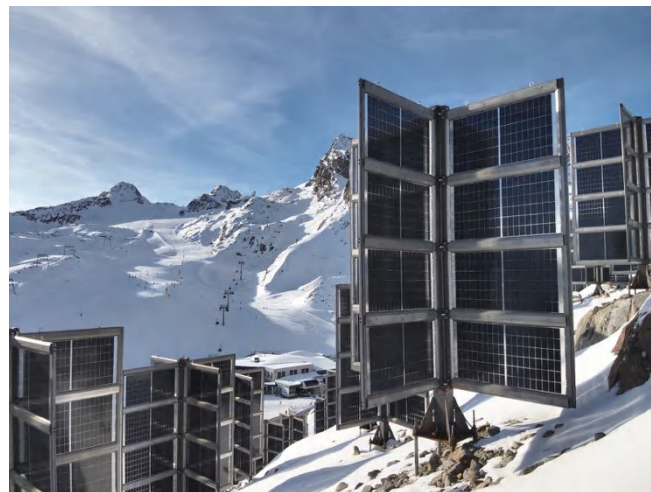
Figure 5: HELIOPLANT® PV-System Tiefenbach Glacier Sölden, Tyrol Austria.
