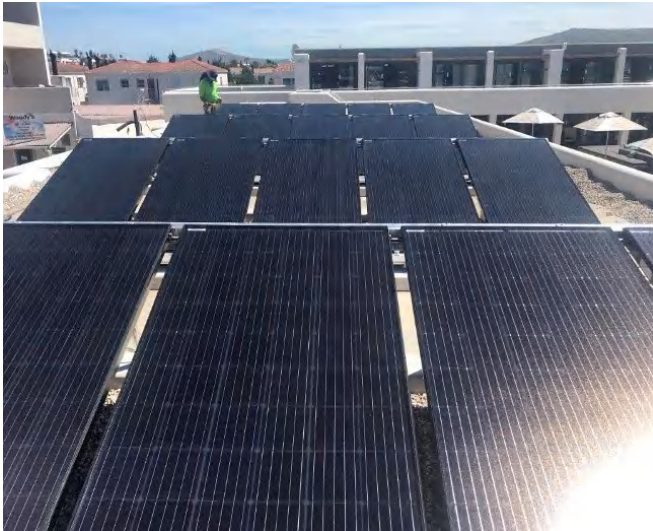
Figure 51: Photo taken by David Volkwyn, Greenline Africa Windtown Langebaan PV-T installation + HP + Tanks. System operating since mid-December 2021; picture taken at 2:30 PM on 25/01/2022, 20 PVT system is generating 69°C and 2000L tank is heated up to 60°C using 20 PVTs.
