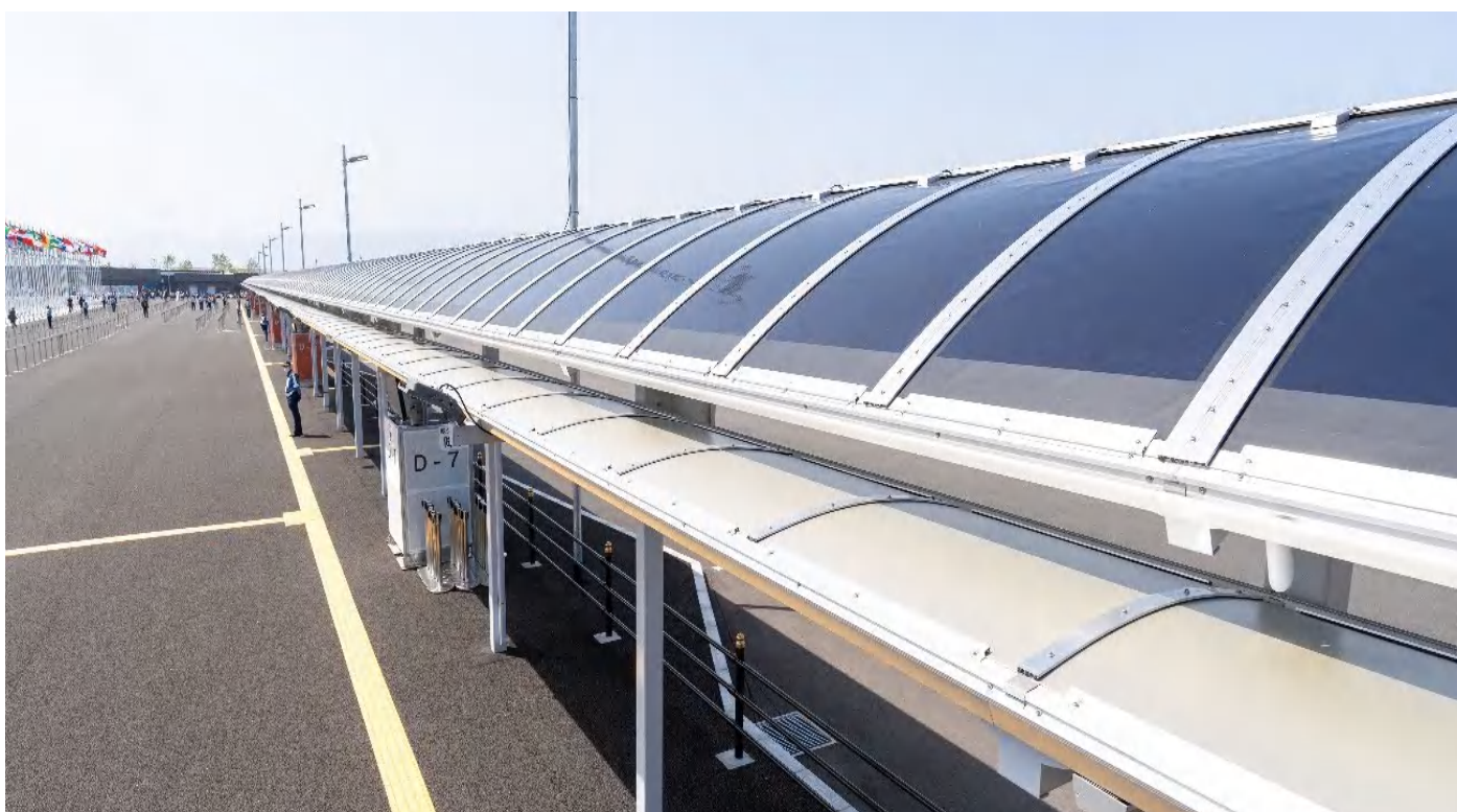
Figure 26: PV system at the Yumeshima Transportation Terminal 1, EXPO2025 OSAKA,KANSAI (Sekisui Chemical Co., Ltd.; film-type perovskite solar cells), (Osaka City, Osaka Prefecture, Japan). © New Energy and Industrial Technology Development Organization (NEDO Green Innovation Fund website).
